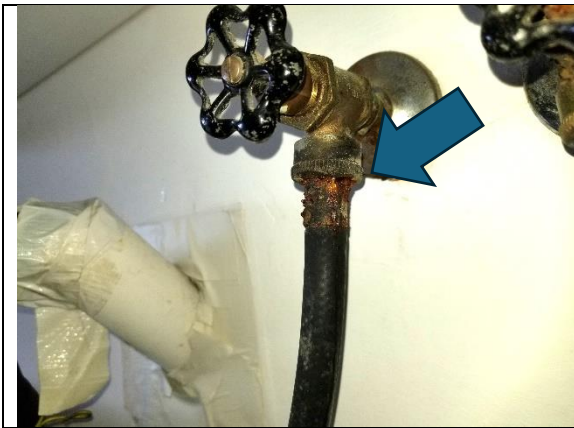
Corrosion at a Washing Machine Supply Hose Connection
