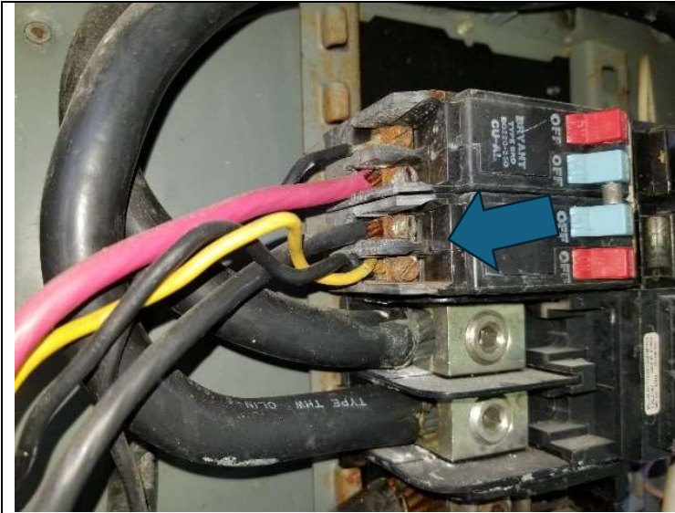
Double Tap - Two Wires at Breaker (Breaker also has less common failure or corrosion damage)
