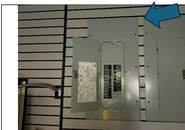
Panel Installed Over a 1 Inch Thick Slat Board (Gaps Between Panel and Breakers)
