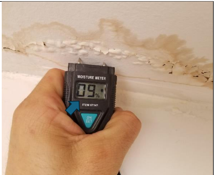
Ceiling Moisture Reading 09% Dry: Lower than the 20% moisture threshold used to gauge gypsum board as "wet"
