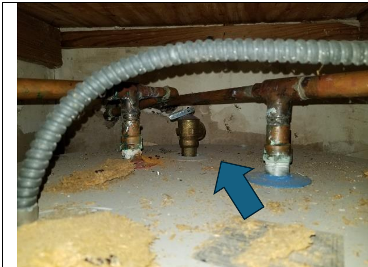
TPRV was Never Connected to a Drain Line
