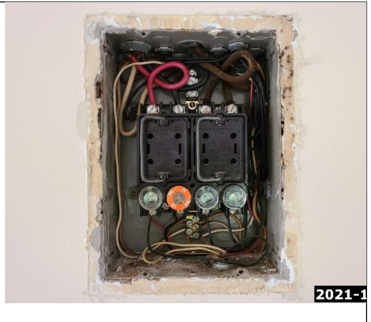
Fuse Subpanel Being Used
