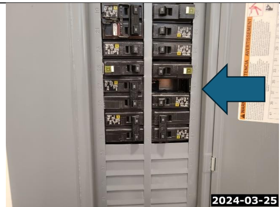
Open Breaker Socket at Panel (Repaired Easily with Clip-In Panel Blank)
