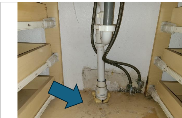
Cabinet Damaged from Leak
