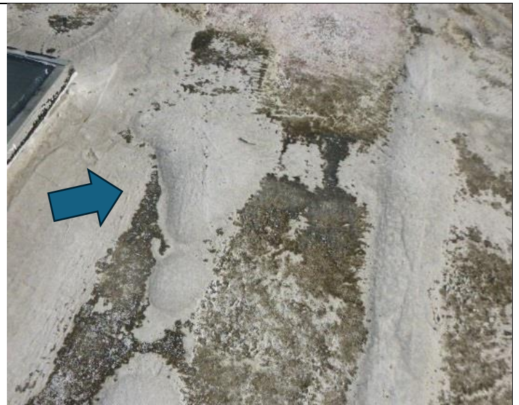
Air Bubbles Under Material This Roof has an Aging Sealant that Failed
