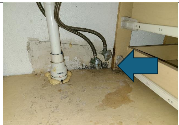
Wall Damage from Leak Moisture
