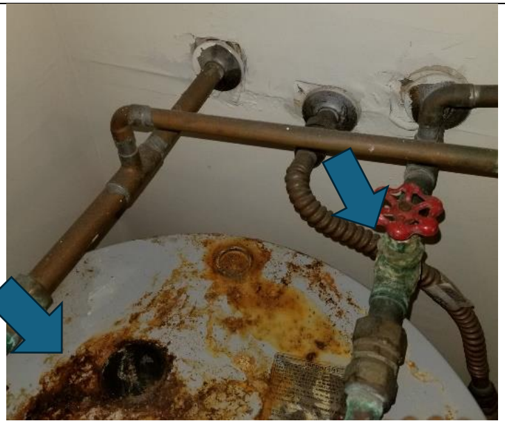
Leaking at Plumbing Valve Causing Rust at Water Heater
