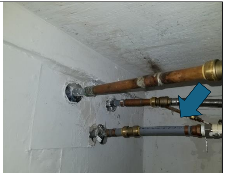
Polybutylene Plumbing (Note Gray Color)
