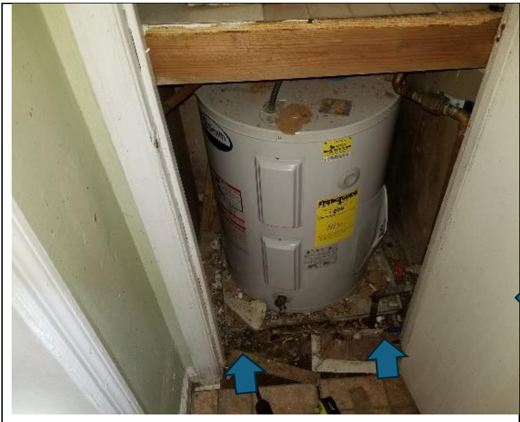
Water Damage at Water Heater Closet Caused by Relief Valve
