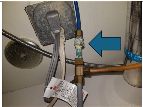
Corrosion at a Supply Line Connection Under a Sink
