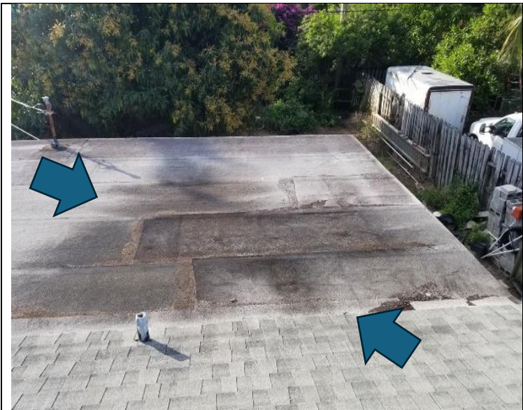
Granule Deterioration and Debris Buildup Typical Signs a Roof has “Ponding” Water
