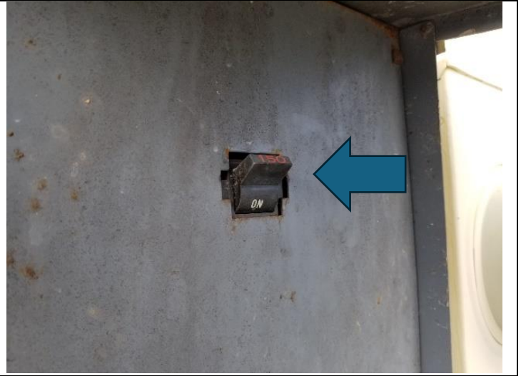
FPE Panel – Breaker Design a Sign of Manufacturer (Red Font)
